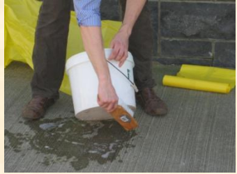
16. Disinfect outside of bucket
